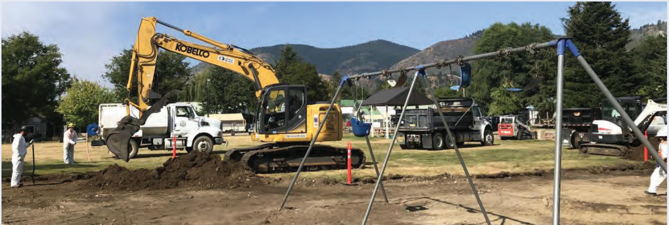
EPA and its contractor excavate and remove lead contaminated soil at Lyn Kaste Gould Memorial Park
