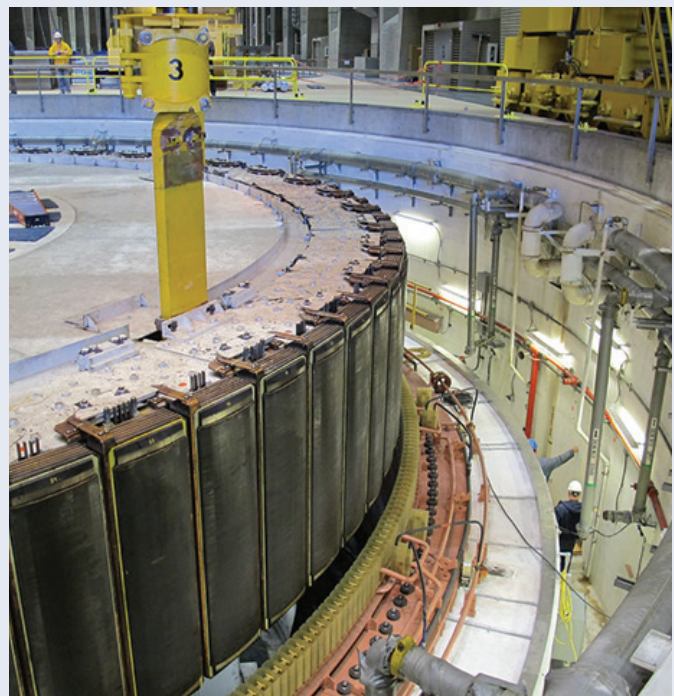
Generator at Grand Coulee Dam
