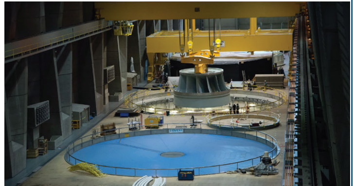
Refurbished turbine runner ready for installation
