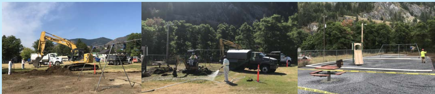
EPA and its contractor excavate and remove lead-contaminated soil at the Lyn Kaste Gould Memorial Park in the town of Northport.
